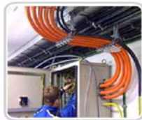
The separation of data and electrical power cabling must comply with safety codes.
