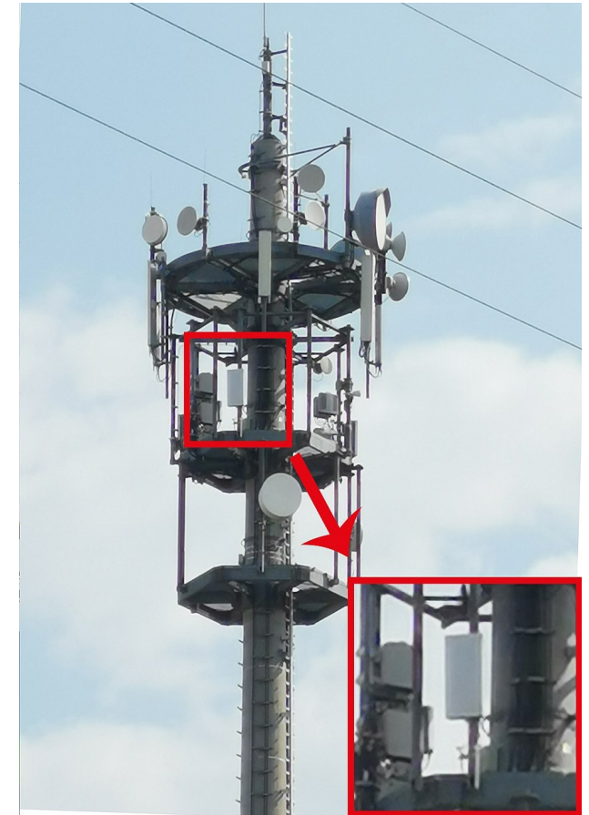
5G 3.5 GHz Cell Site of Vodafone in Karlsruhe, Germany
