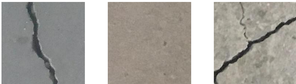
Figure 18: Concrete crack images dataset
